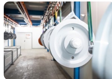
New drying facility with waste heat recovery
