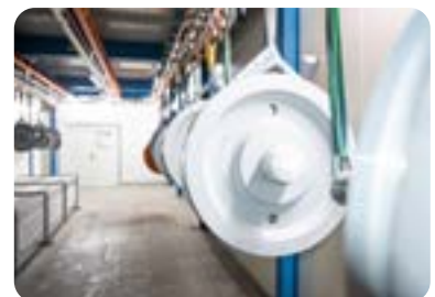
New drying facility with waste heat recovery
